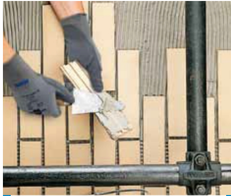
Exterior laying of strip tiles. N.B. Completely fill all lugs and ribs
