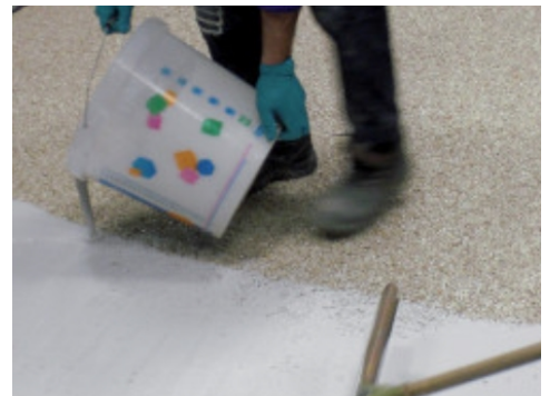
Application of Ultratop on the hardened surface of the mixture made of natural aggregates + Mapefloor 910
