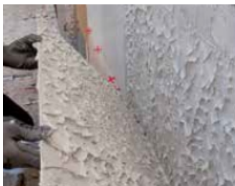
Checking the back face of the tile if it is completely buttered when laying on an external façade
