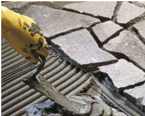
Installation of external hewn back stones with or without buttering, depending on thickness and size
